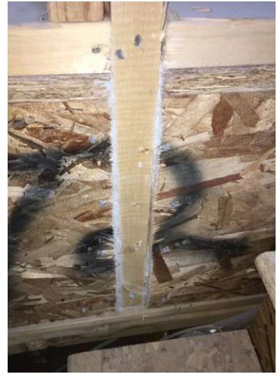
Rim joist gaps
