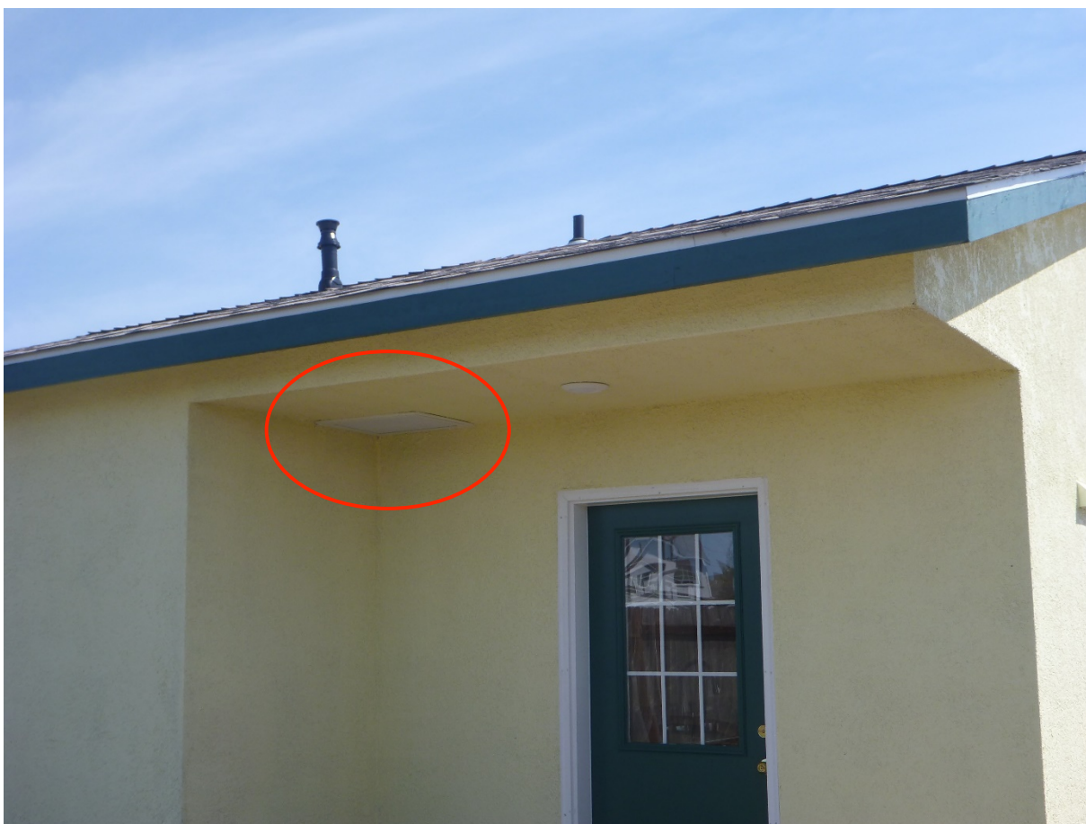
Figure A3.34 Fresh Air Intake in Back Porch Ceiling (Chitwood Energy Management)
