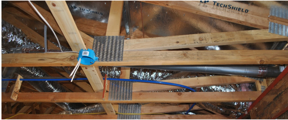
Figure A3.42 Electrical Box for LED Fixture (Chitwood Energy Management)
