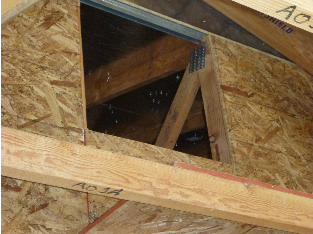
Figure A3.15 Attic Access Does Not Penetrate the Ceiling Insulation (Chitwood Energy Management)
