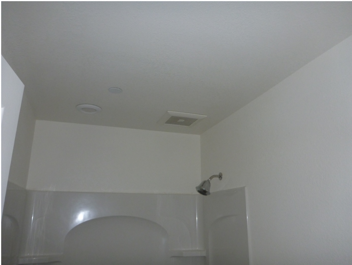
Figure A3.35 Bath Exhaust Fan (Chitwood Energy Management)
