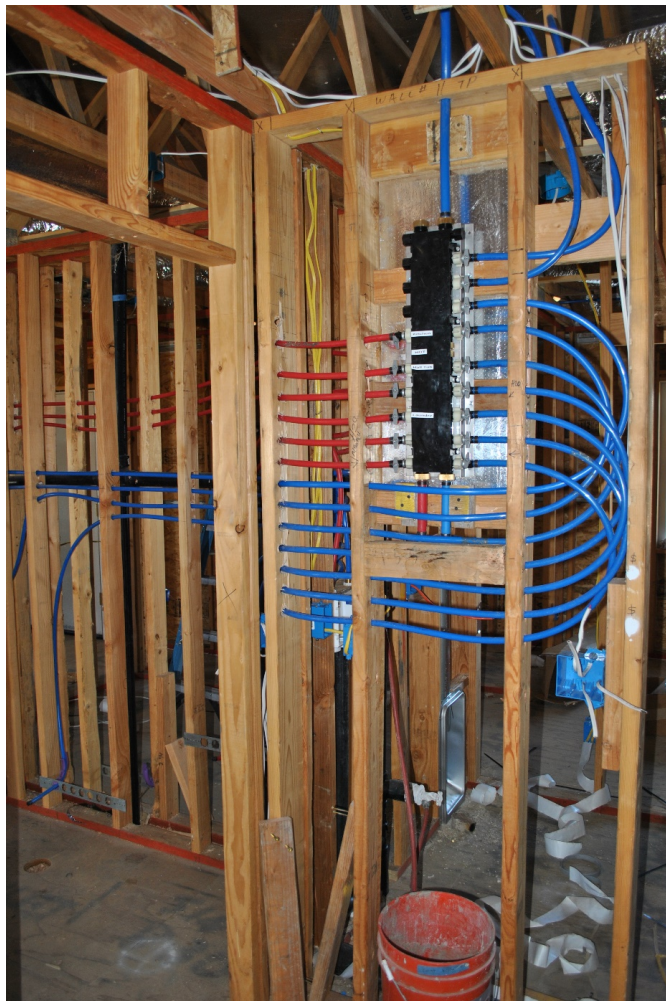
Figure A3.41 Manifold Water Distribution System (Chitwood Energy Management)
