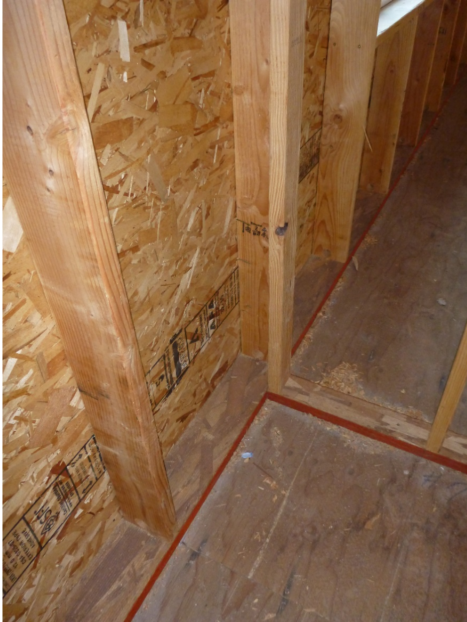
Figure A3.13 No Extra Framing at Wall Intersections (Chitwood Energy Management)
