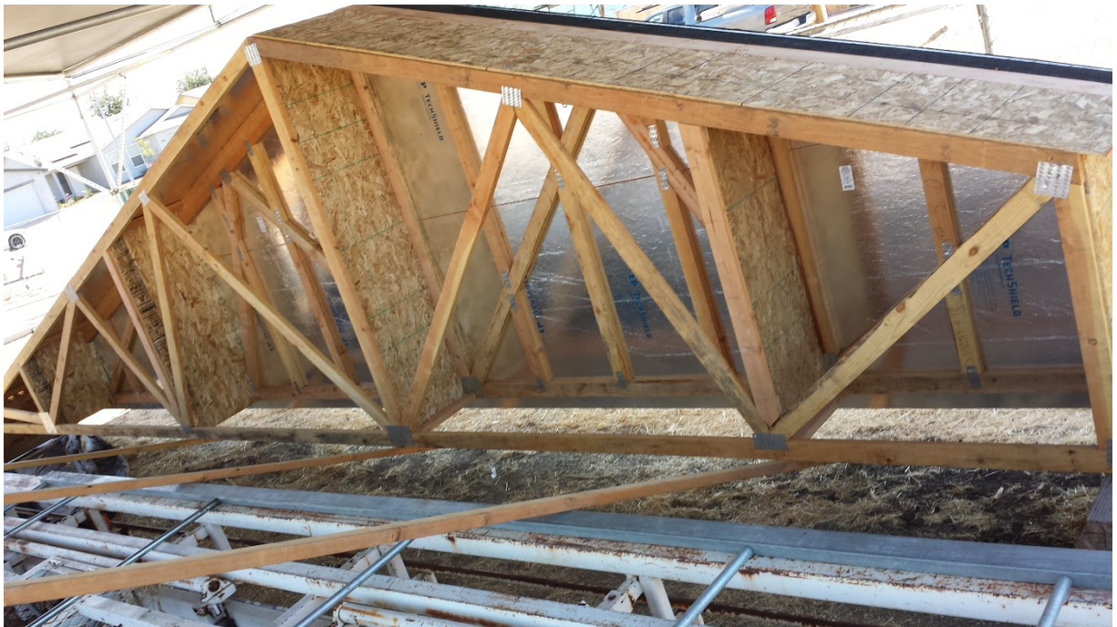
Figure A3.19 Gable End Trusses Built on the Ground (Chitwood Energy Management)
