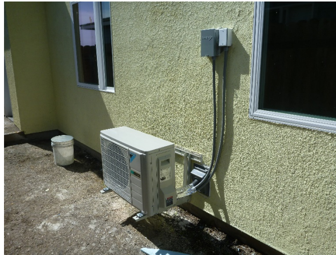
Figure 12. Installed Heat Pump (Chitwood Energy Management)
