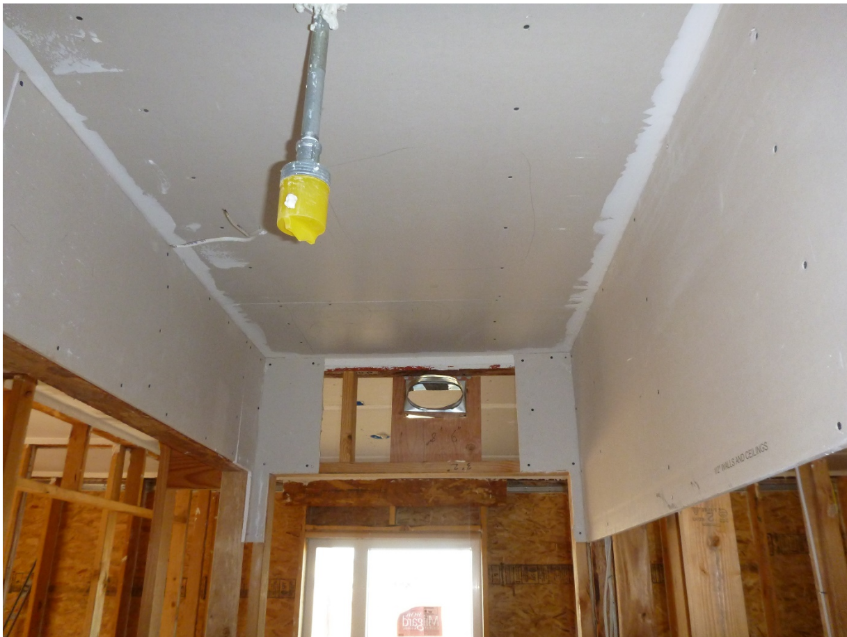
Figure A3.37 Ducts in Conditioned Space (Chitwood Energy Management)
