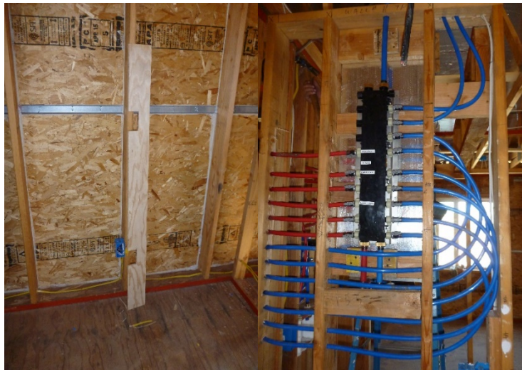
Figure A3.11 Installed Plumbing (Chitwood Energy Management)
