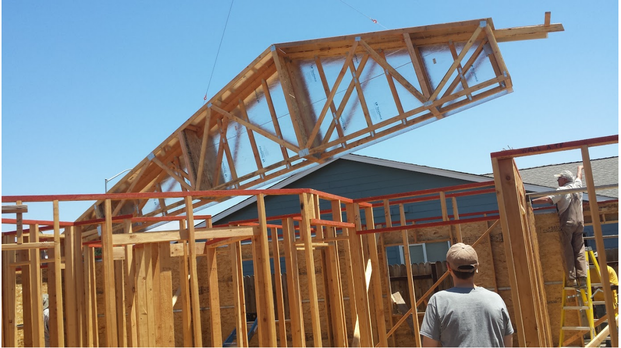
Figure A3.20 Gable End Trusses Being Craned into Place (Chitwood Energy Management)
